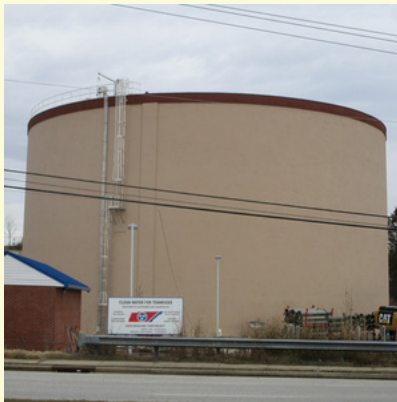
Storage Tank (1) 5 Million Gallon Storage Capacity
