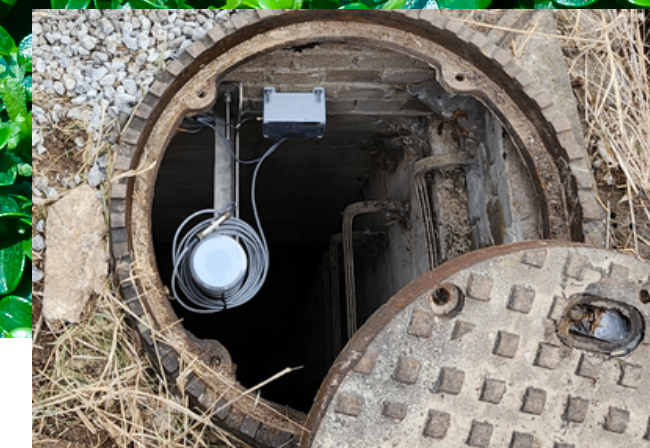
Flow Monitoring Unit
